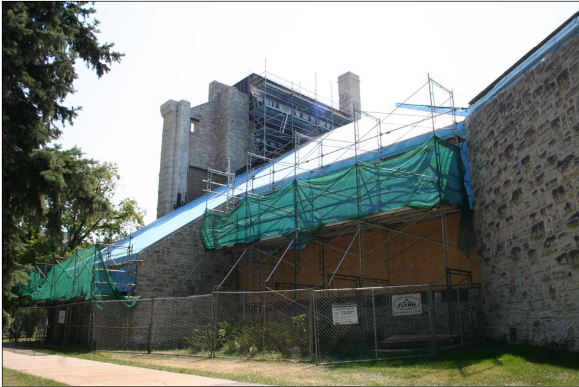
Plate 34 – St. Boniface Cathedral, 190 Avenue de la Cathédrale, work on the roof, 2012. ( M. Peterson, 2012. )
