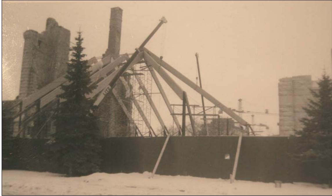
Plate 5 – Construction of the new Cathedral building, December 1971. ( Courtesy of St. Boniface Parish Office. )
